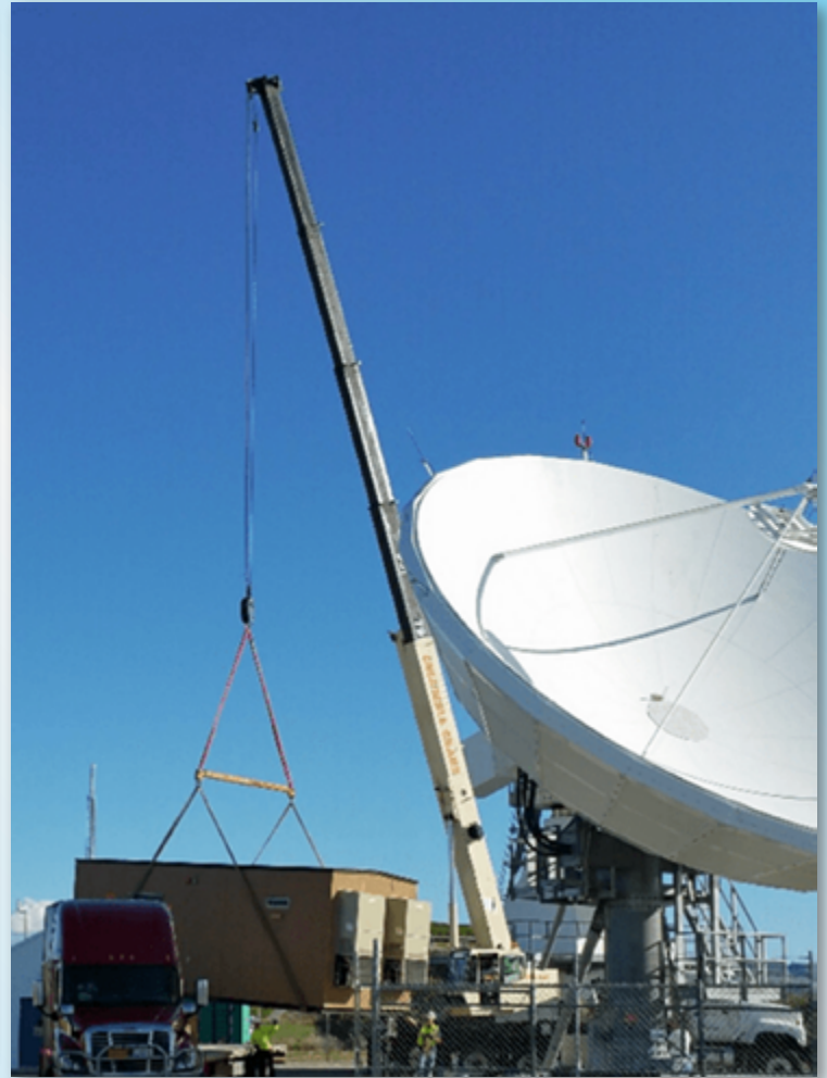
The new service shelter being installed next to the WAAS Uplink Antenna at Brewster, Washington.
