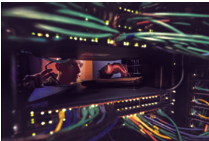
Air Force Airman 1st Class Thomas Schoening, a cyber transport systems airman, stands in the server room at the 153rd Airlift Wing, Wyoming Air National Guard Base, Cheyenne, Wyoming, in November.
