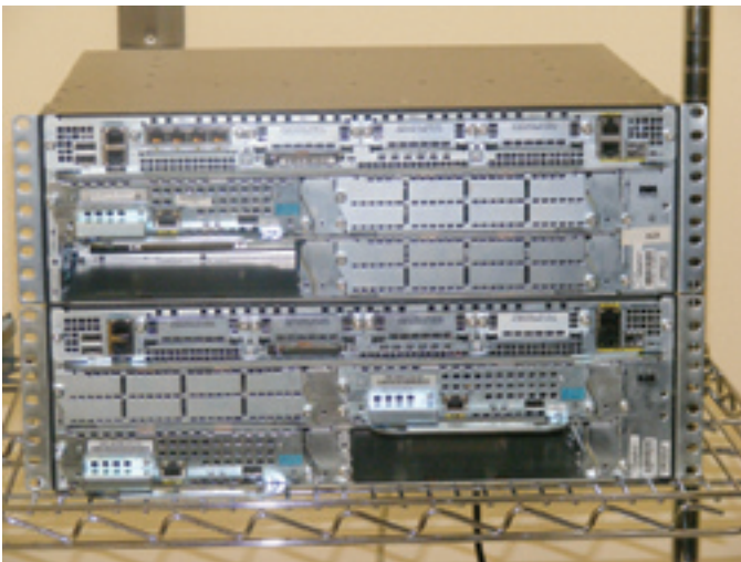
The SkipWare AXP installed in a pair of Cisco 3845 ISRs, both as a standalone PEP (top) and with a WAAS module (bottom)
